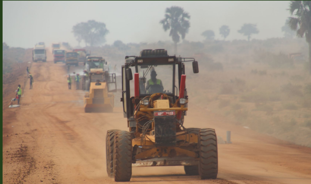
Road construction work in Murchison Falls National Park. Image credit: LoneExplorer, Uganda.
